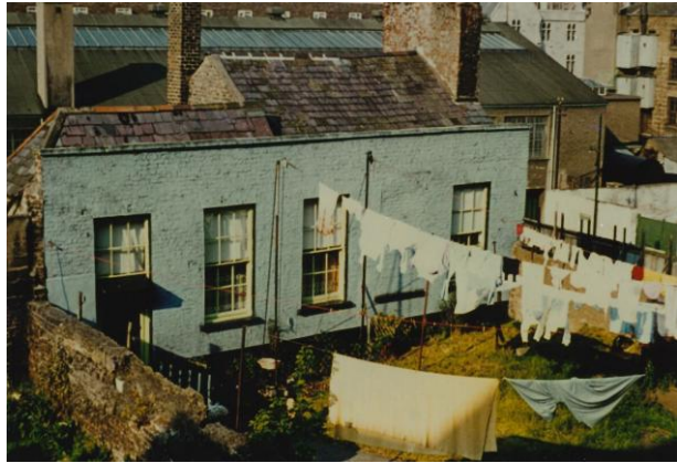
View of upper ground floor of former L-shaped mews building at rear of 4 Henrietta Street which was burnt down in 1985. Gable walls and floor survive of upper ground floor and supporting vaults of lower ground floor survive. Note large chimneystack on east gable on RHS.
