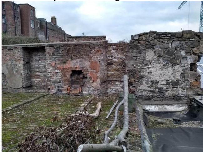
View of surviving central gable wall of former mews building with remains of small fireplace & cupboard recess.
