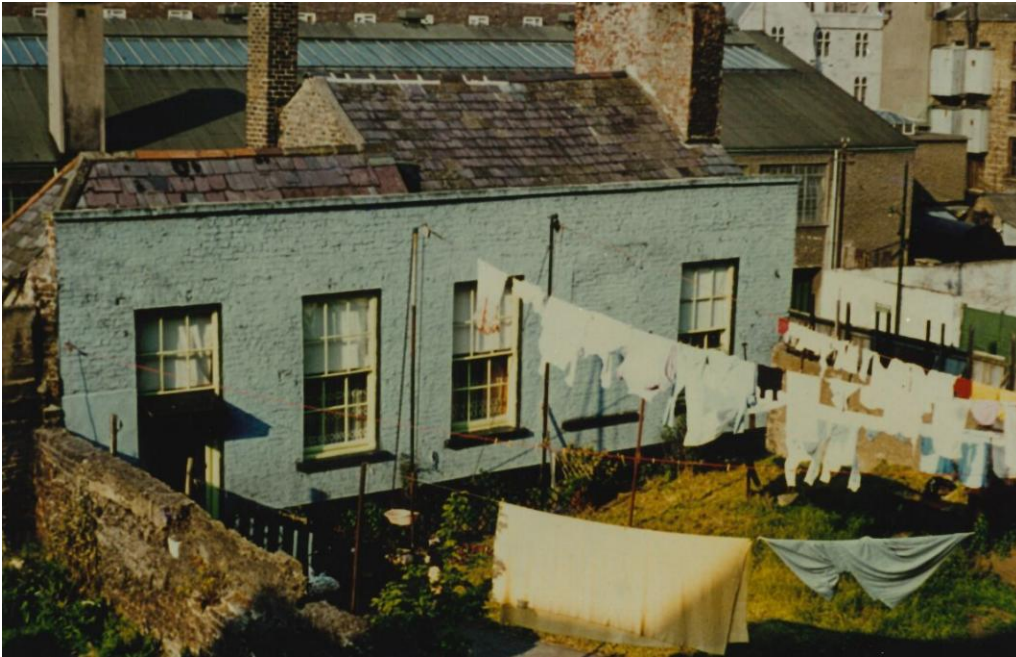
View of upper ground floor of former L-shaped mews building at rear of 4 Henrietta Street which was burnt down in 1985. The gable walls and side boundary walls still survive.
